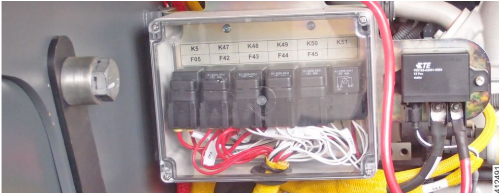
Fuses in engine compartment
