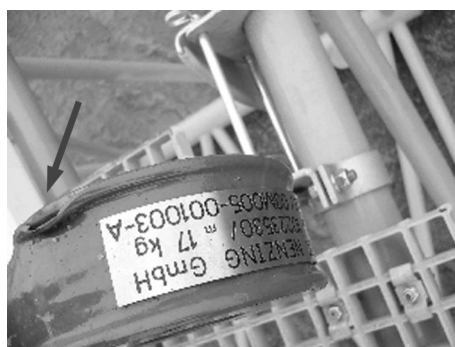
Fig. 5939: Damage to the protective sheath
