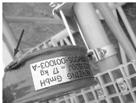
Fig. 6030: Damage to the protective sheath
