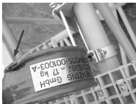
Fig. 3463 Damage to the protective sheath
